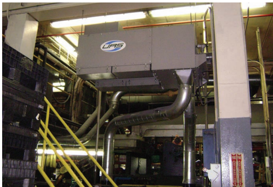
A cartridge dust collector hangs from the plant's ceiling above a roller mill and provides clean cooling air to the mill's two fan-cooled motors.
